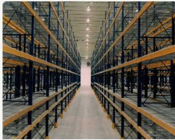
Selective Pallet Racking
